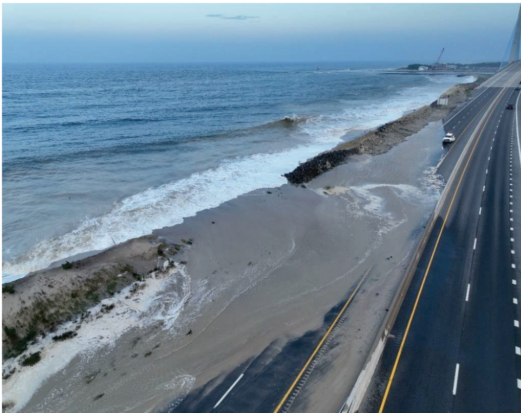
Figure 3. August 17, 2024. View of the dune breach at Delaware Seashore State Park (looking south). The SR-1 northbound lane is covered in water and sand, forcing a road closure.
