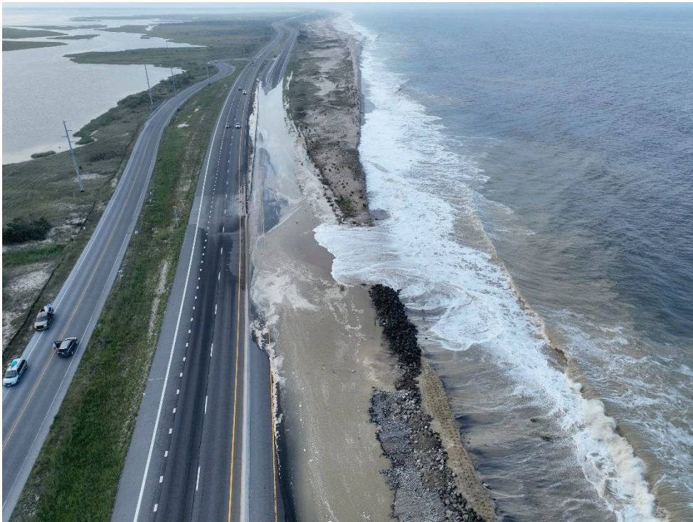
Figure 2. August 17, 2024. Aerial view of the dune breach at Delaware Seashore State Park (looking north). The SR-1 northbound lane is closed to vehicles and completely covered in ocean water, sand, and debris.
