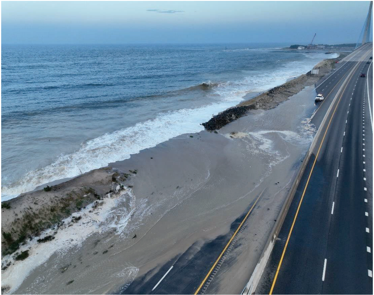
Figure 2. August 17, 2024. View of the dune breach at Delaware Seashore State Park (looking south). The SR-1 northbound lane is covered in water and sand, forcing a road closure.
