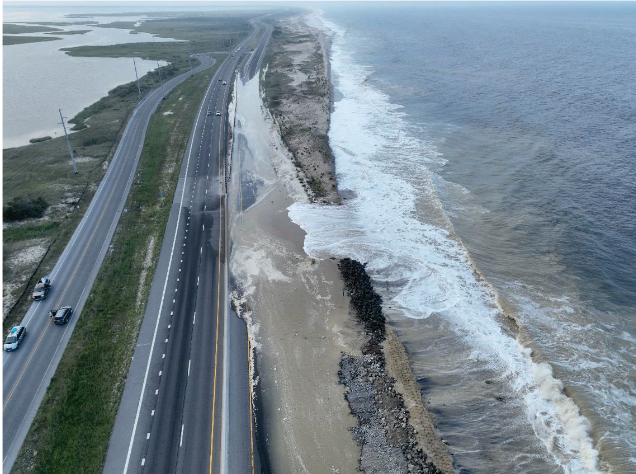
Figure 1. August 17, 2024. Aerial view of the dune breach at Delaware Seashore State Park (looking north). The SR-1 northbound lane is closed to vehicles and completely covered in ocean water, sand, and debris.
